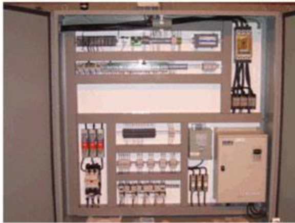
Figure 1, Steel Processing Machine Control Panel
